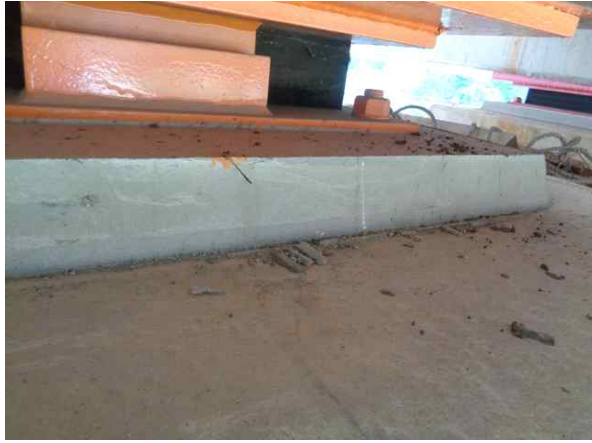
P2-Sh10 무수축물탈 균열(0.1mm/0.2m)
